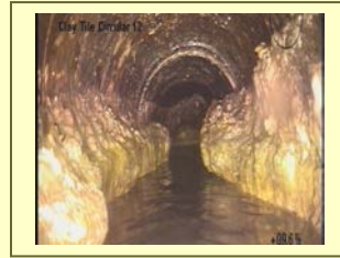
The lack of maintenance can lead to clogged sewer pipes.
